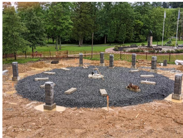
Construction progress on June 22, 2021 shows stone base and concrete bases for the eleven six-foot-high granite panels and fence pillars.
